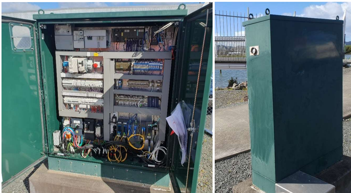
Figure 2-6: Electrical switchboard internal space limitations
