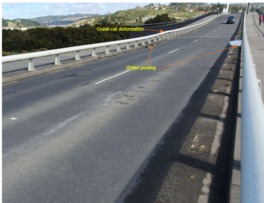
Figure 2-11: Water pooling and the pavement settlement
