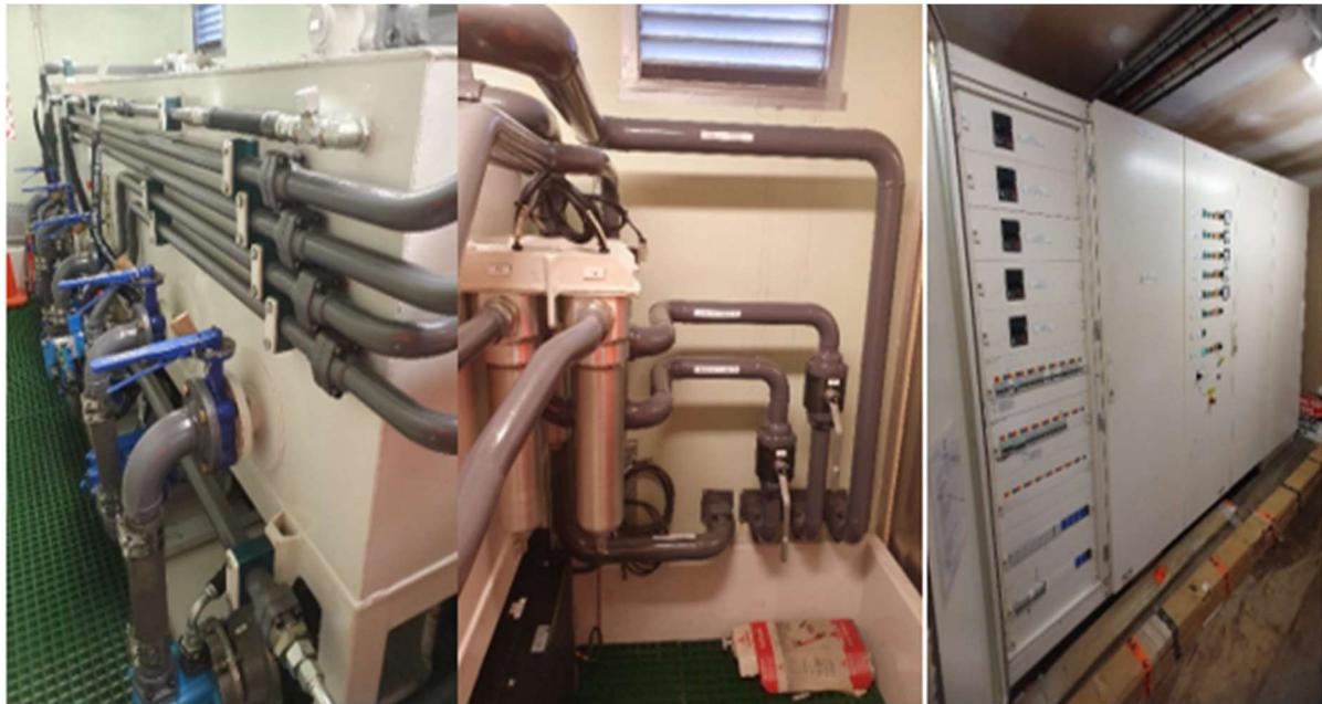
Figure 1-3: Hydraulic & Electrical plant room
