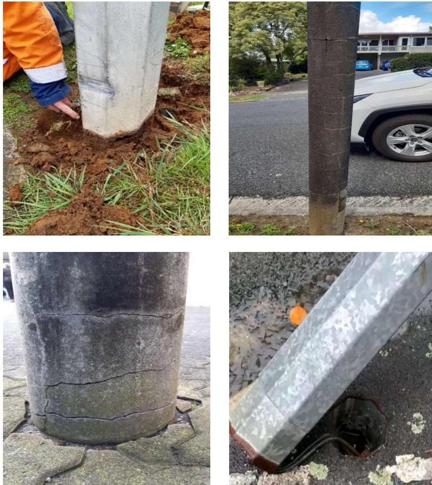
Figure 1-6: failures of steel and concrete streetlight columns
