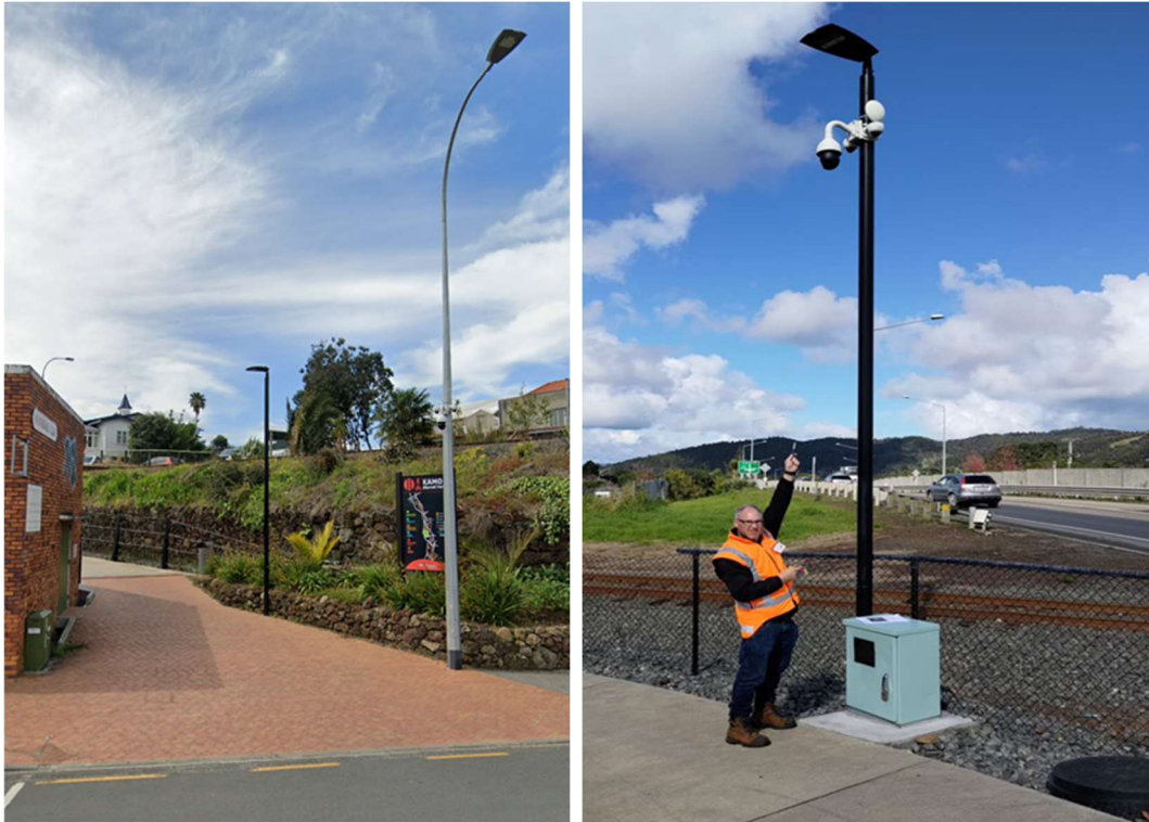
Figure 1-4: CCTV cameras installed in Kamo Shared Path (KSP) on streetlight poles
