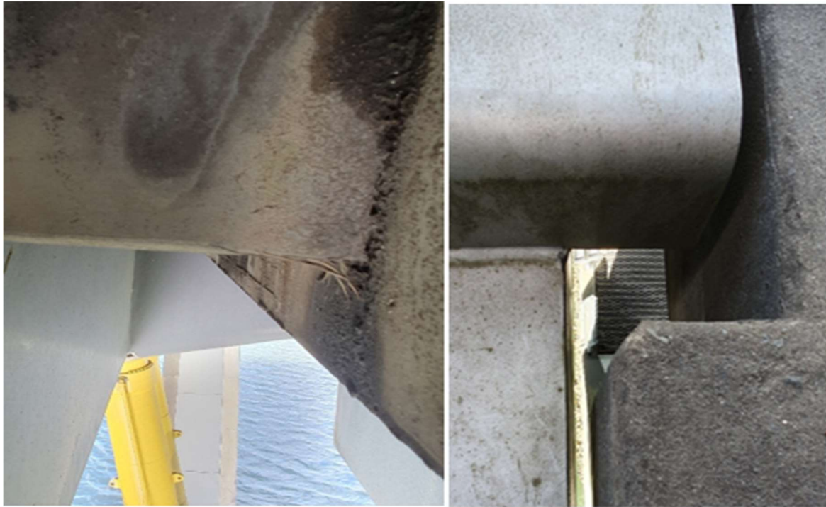
Figure 2-13: Gap between the bridge lifting section and fixed portion and water tracking marks on the piers
