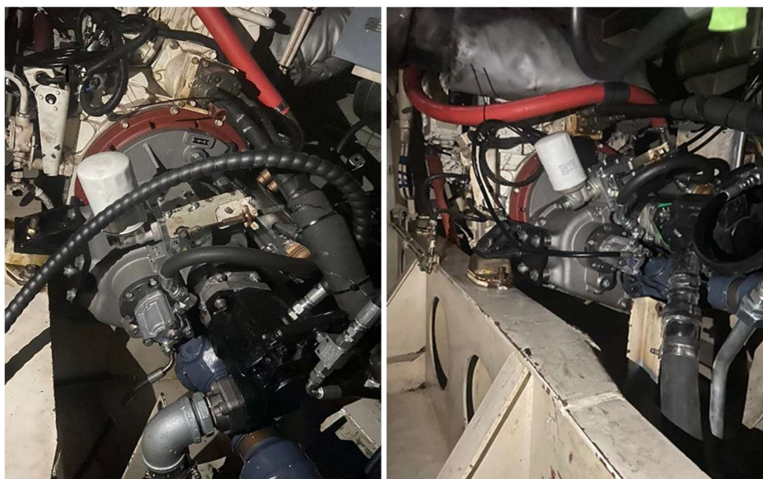
Figure 1-2: Newly installed gearboxes units
